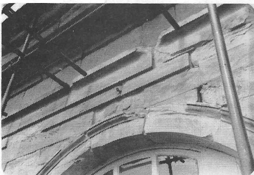
Window arch and stringcourse above, with spaces where the masonry has crumbled
