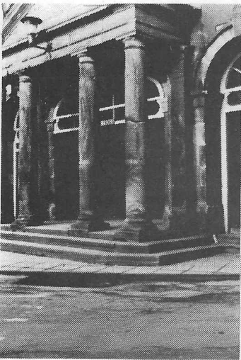
Weathering has scarred the columns of the portico and widened joints between the blocks
