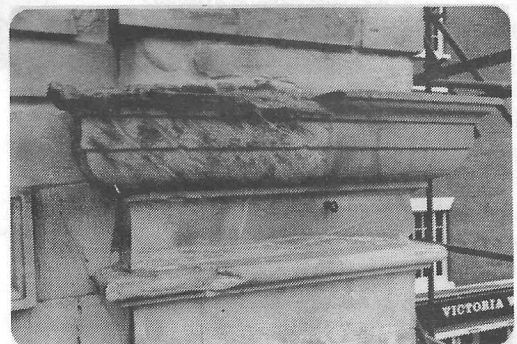
This and other parts of the cornice are badly decayed
