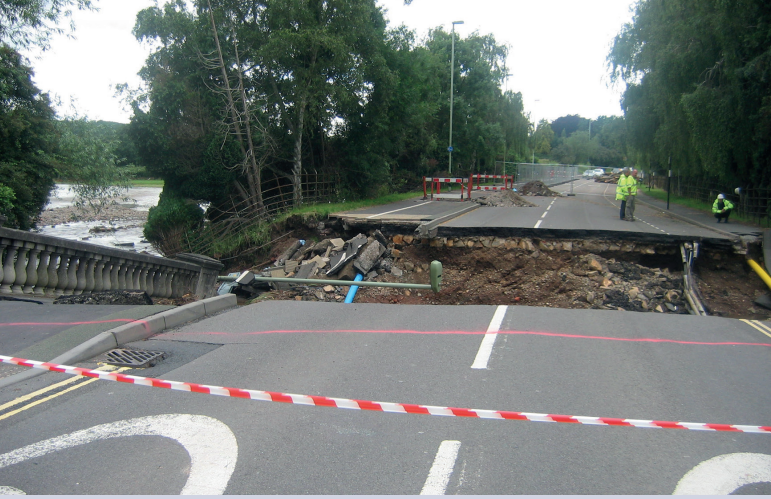
2007: collapse of Burway Bridge, and Coronation Avenue
